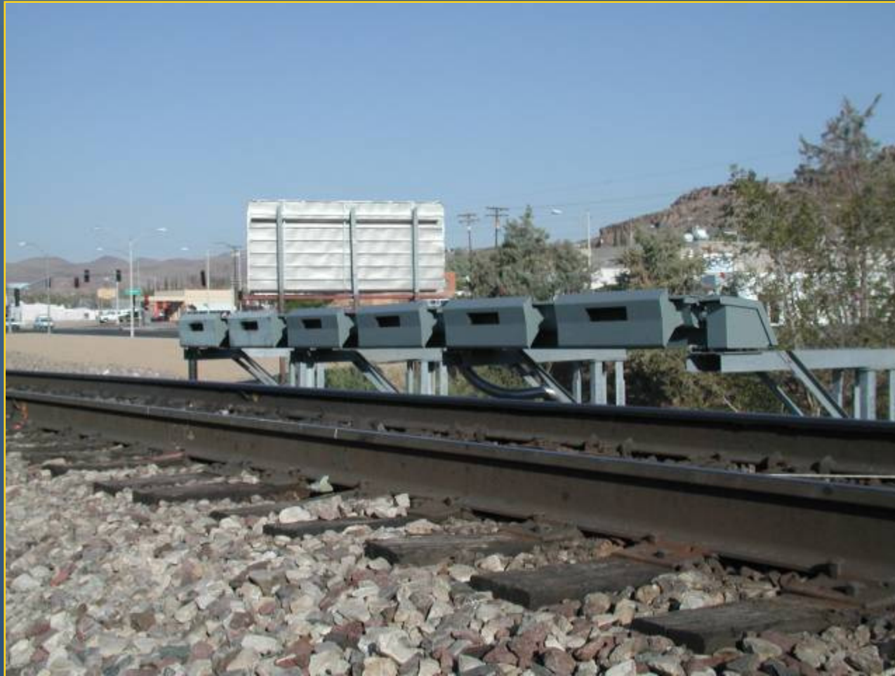
Trackside Microphone Array
