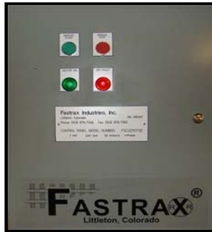
FSC2210732 CONTROL PANEL
