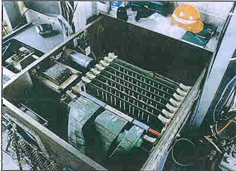
Figure 5-20: Unit 1 microprocessor mainframe top view
